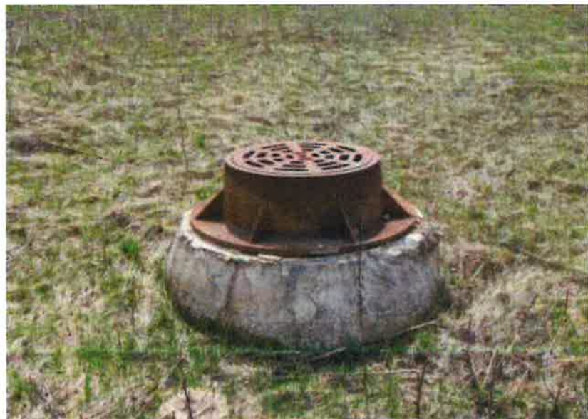
Pond I.D. #SWP02s001 Secondary basin outlet
