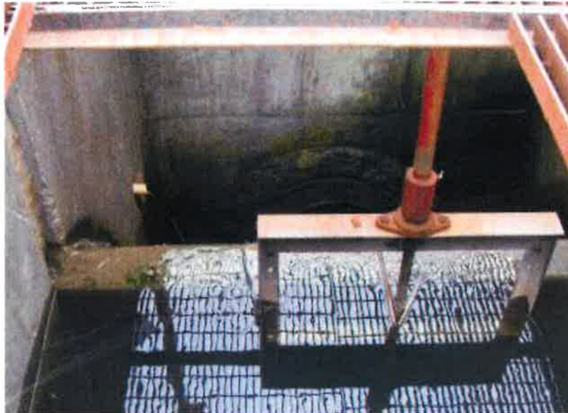
Pond I.D. #SWP02s002 Outlet control structure
