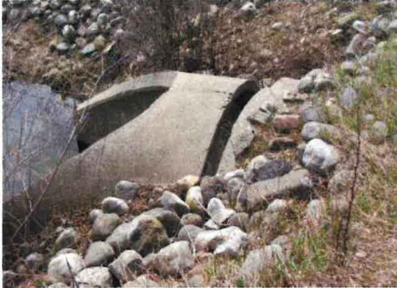
Pond I.D. #SWP02s002 Disconnected 72" outfall
