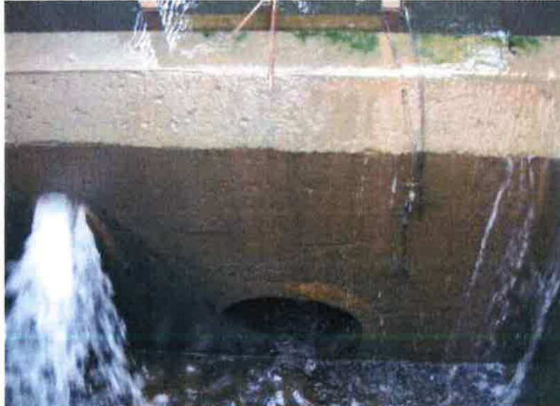
Pond I.D. #SWP02s002 Outlet control structure.
