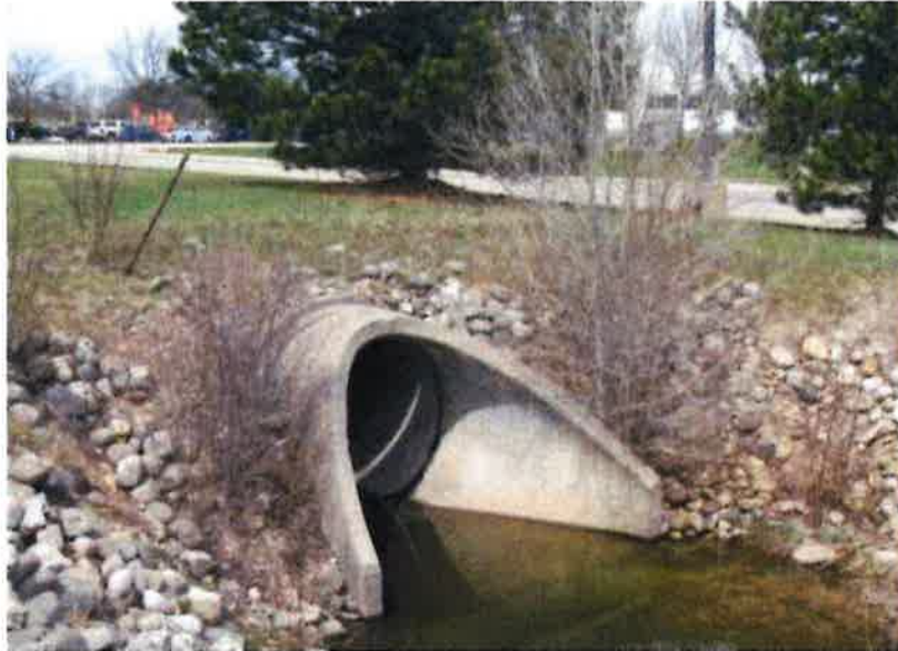
Pond I.D. #SWP02s002 Woody vegetation by 72" outfall
