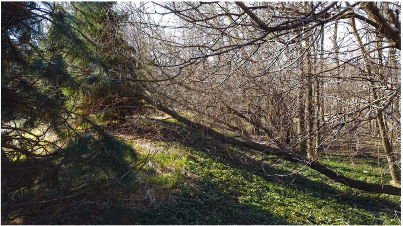
Pond SWP3N001 – Numerous trees have fallen along the Northern berm near the Emergency Spillway
