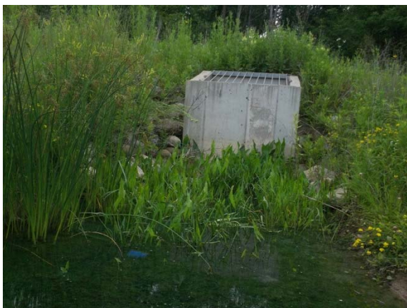
Figure 3: Overview of the Outlet Structure located in the Southeast Portion of the Pond, Looking to the Southeast
