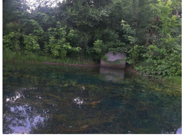
Figure 4: Overview of Outlet Structure located on the Southeast Portion of Pond, Looking East
