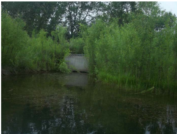
Figure 3: Photo of Outlet Structure Located on the Northeast Portion of the Pond
