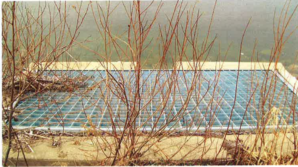
Overflow Structure ST23N021
