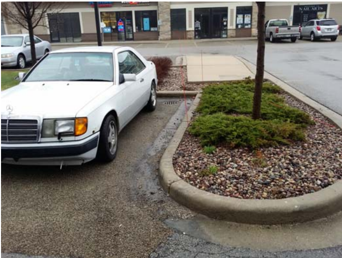
Photo #4: Porous pavement in north parking field of west building. Minor surface wear visible.
