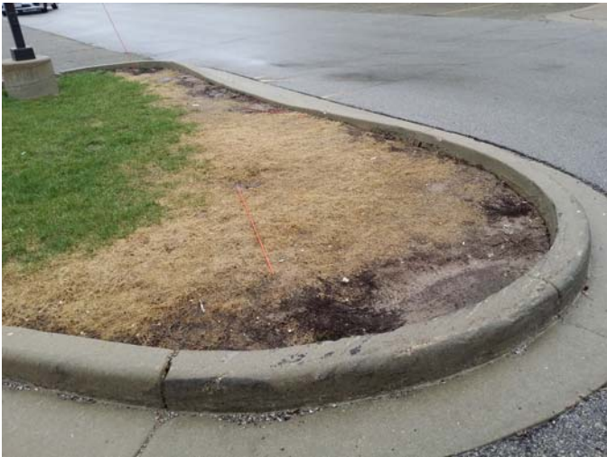
Photo #3: Parking lawn areas showing signs of settlement behind curbs and adjacent to walkways.
