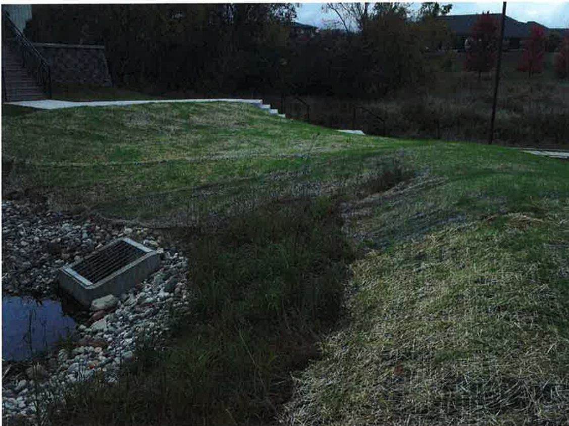
NE of pond, looking west at emergency spillway and outlet structure (Oct. 21, 2013)
