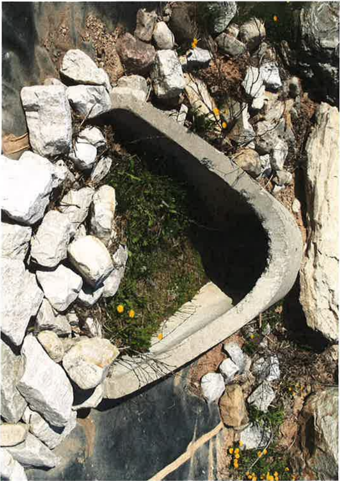
24" inlet pipe to North Pond
