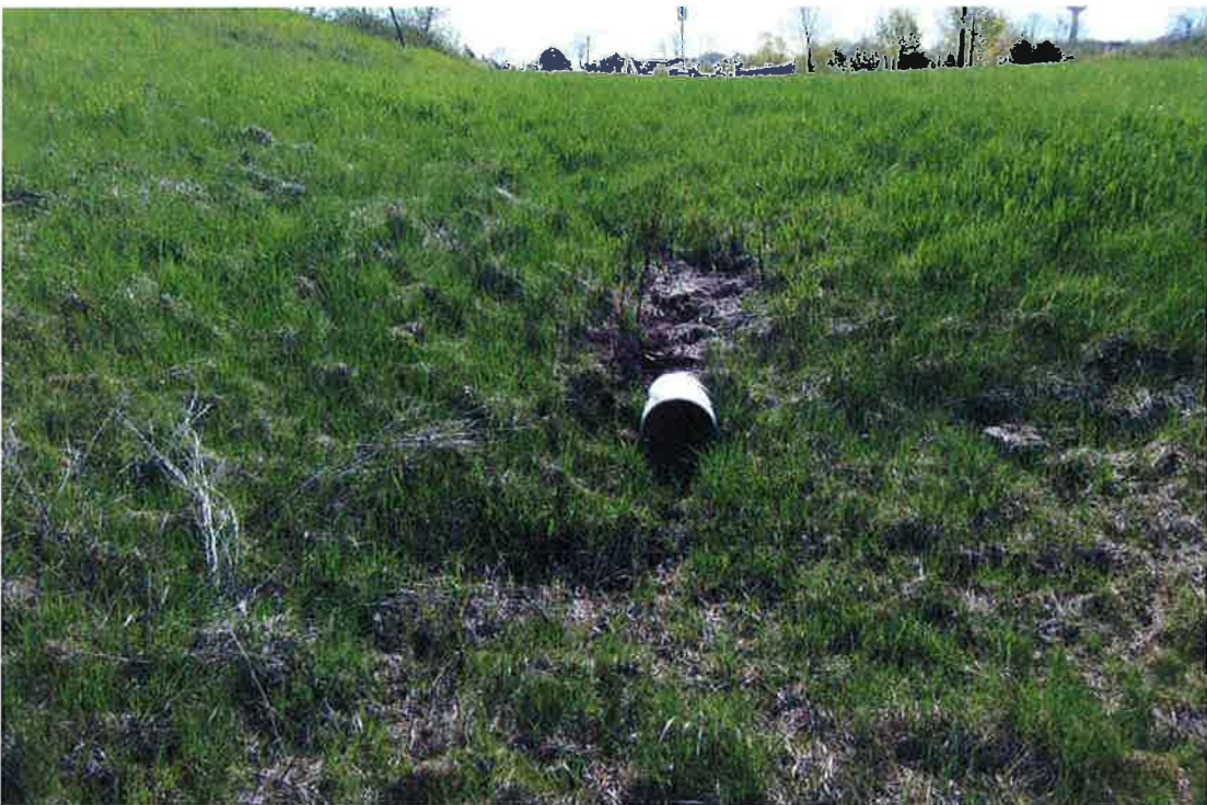
Sediment trap outfall, permanent site storm lateral.
