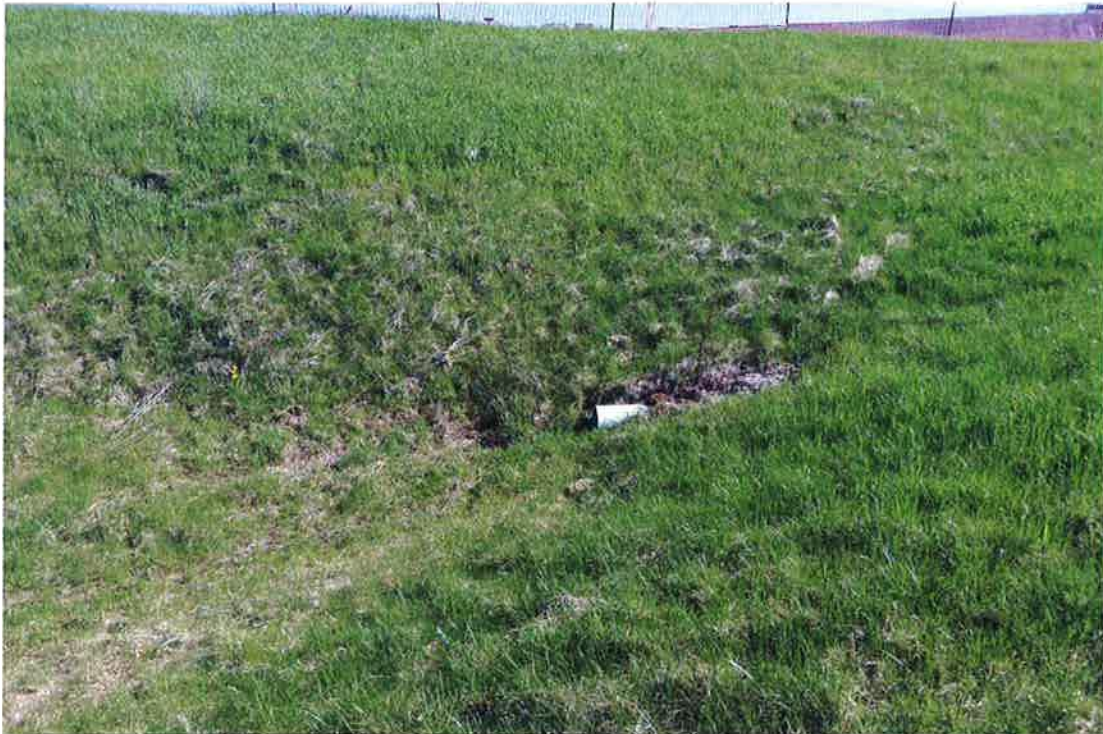
Sediment trap outfall, permanent site storm lateral.
