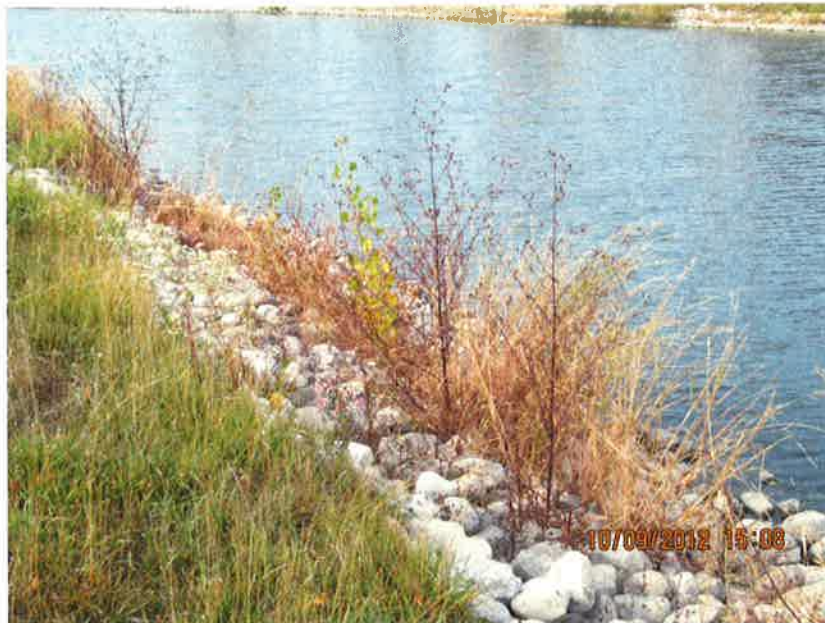
Pond I.D. #SWPO2S002 Woody vegetation along south embankment of pond
