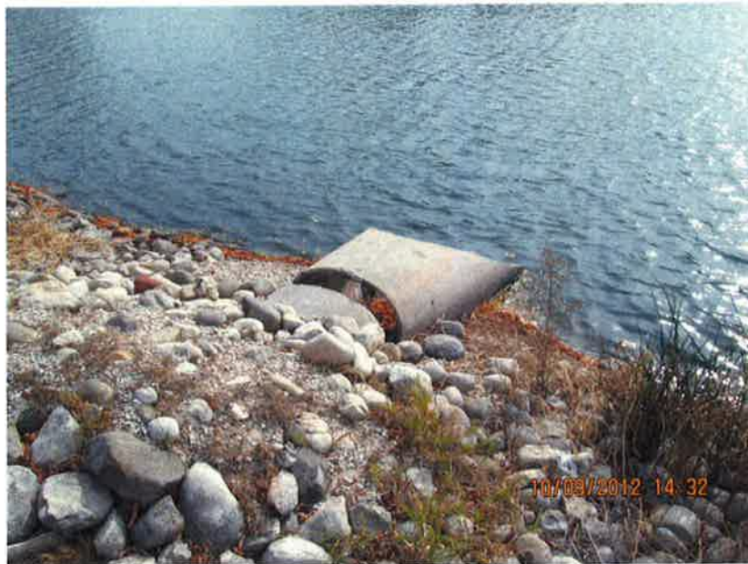
Pond I.D. #SWPO2S002 Disconnected 19-inch x 30-inch outfall to pond
