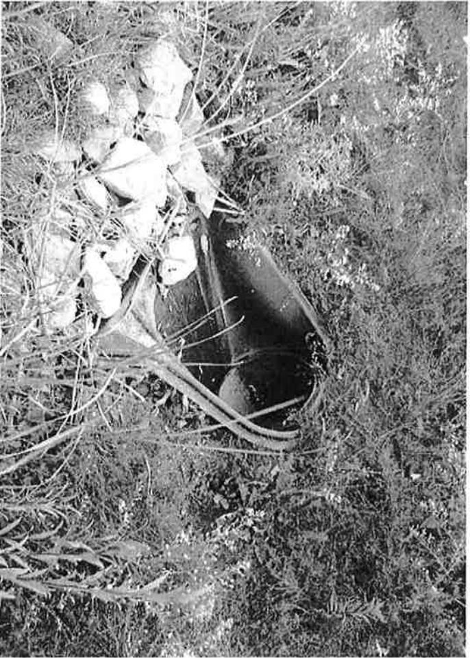
Picture #4 - Inlet Pipe
