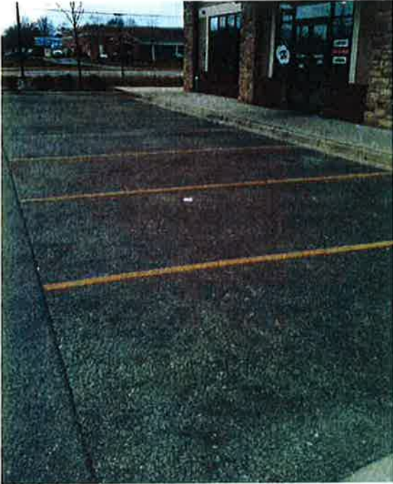
Photo #11: Porous Pavement – looking south at east side of Building A parking area (good condition)
