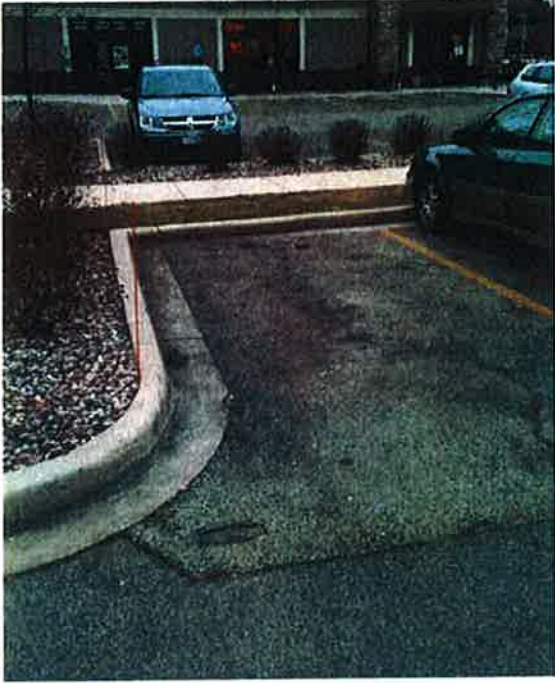
Photo #13: Porous Pavement – looking at the low point in the portion of pavement replaced due to material defect on the north side of the parking area in front of Building A (good condition)
