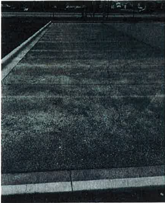
Photo #7: Porous Pavement – looking south at west side of parking area east of Building A (crack mid slab - good condition)
