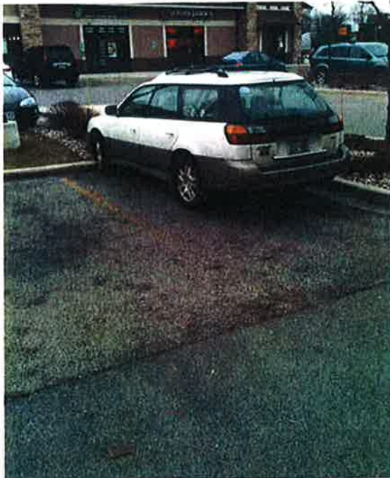
Photo #10: Porous Pavement – looking south at the low point for the area along the north side of the main drive aisle and in front of Building A (good condition)
