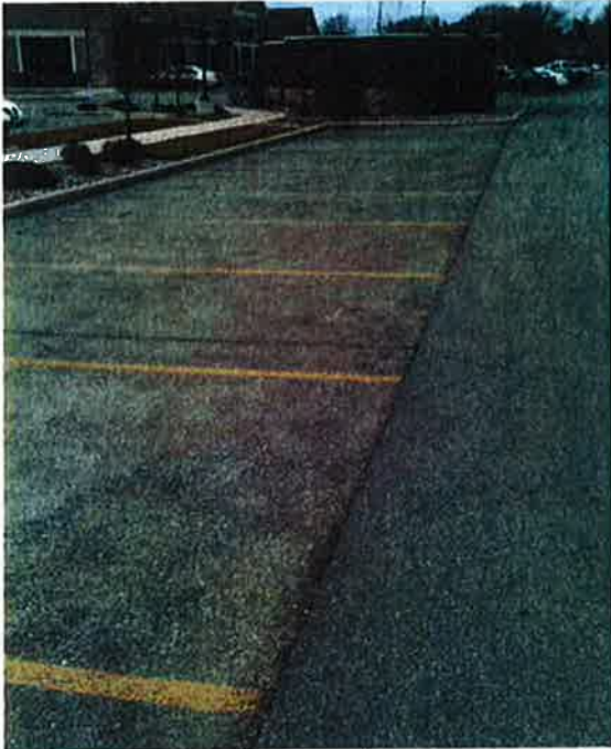
Photo #9: Porous Pavement – looking west at north side of parking area north of main drive aisle and south of future Building B (good condition)
