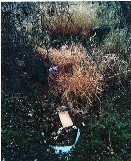
Photo #2: 12" Outfall Structure (looking north at berm opening and unnamed tributary to Lilly Creek)
