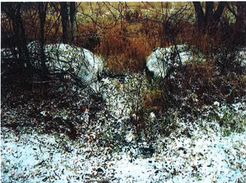
Photo #2: 12" Outfall Structure (looking north at berm opening and unnamed tributary to Lilly Creek)
