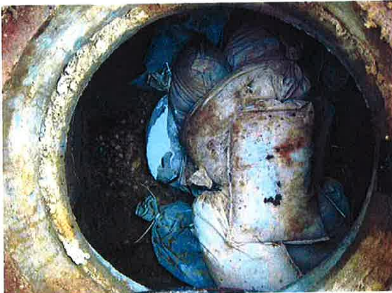
Photo #4: North chamber of outfall structure with sand bag filter (good condition)
