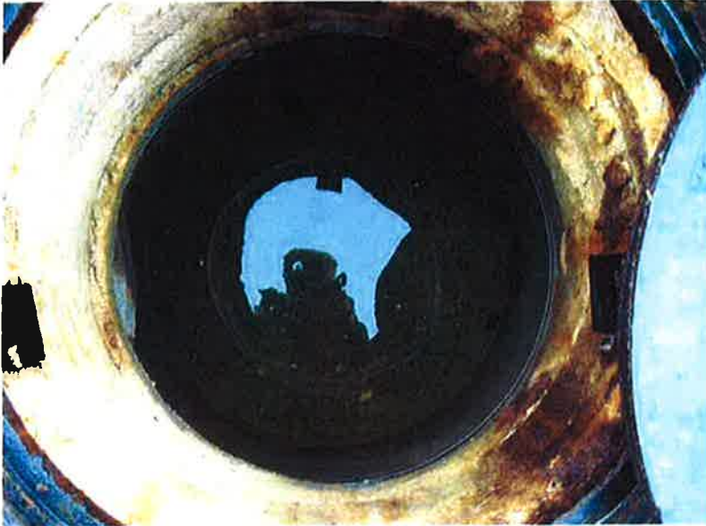
Photo #5: South chamber of outfall structure (good condition – frogs in clear water)
