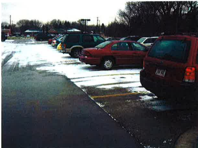
Photo #12: Porous Pavement – looking west at north side of Building A parking area (good condition)
