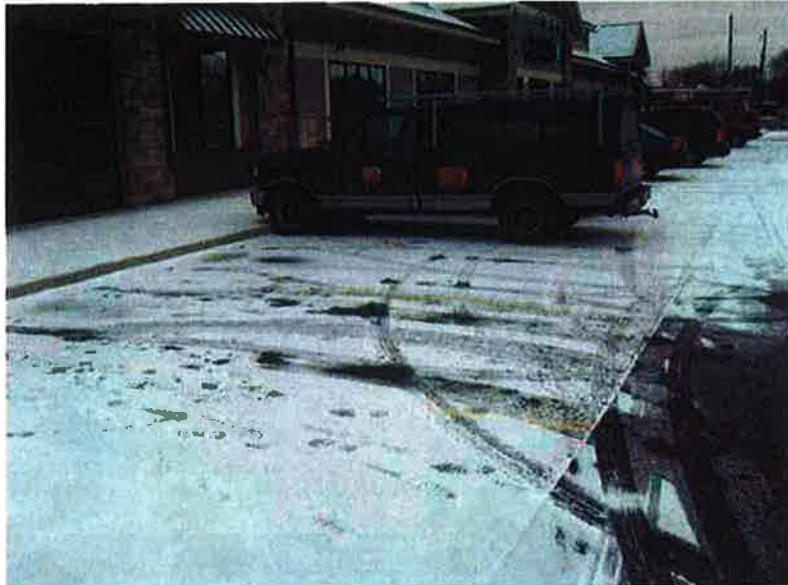
Photo #11: Porous Pavement – looking west at south side of Building A parking area (good condition)
