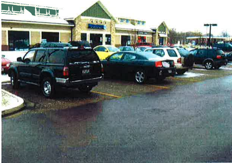
Photo #13: Porous Pavement – looking south at south side of north parking area, north of Building A (good condition)
