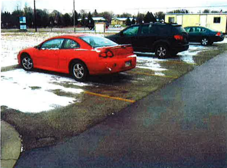
Photo #9: Porous Pavement – looking north at east side of parking area west of Building A (good condition)
