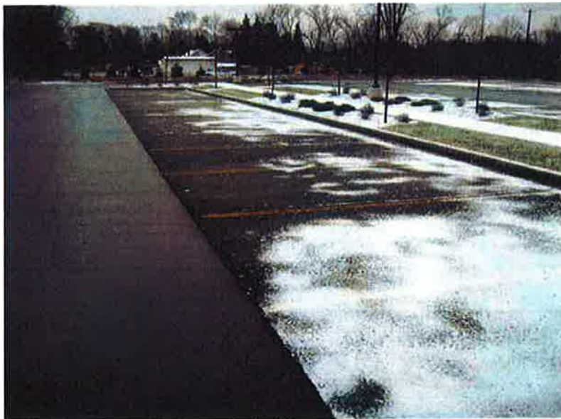
Photo #14: Porous Pavement – looking east at south side of north parking area, north of future Building B (good condition)
