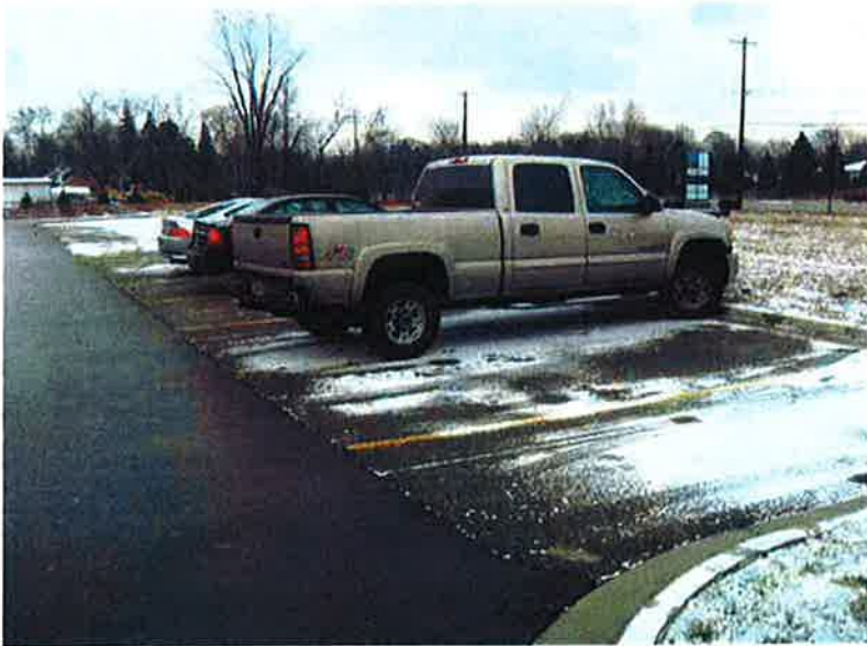
Photo #8: Porous Pavement – looking east at north side of center parking area (good condition)
