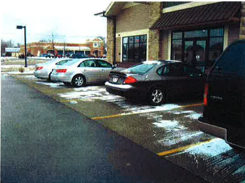
Photo #10: Porous Pavement – looking east at west side of Building A parking area (good condition)
