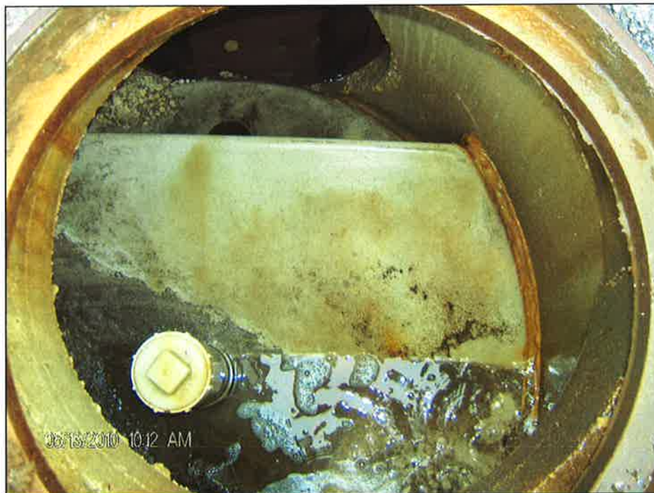
Site Photo 4: May 13, 2010 Stormceptor
