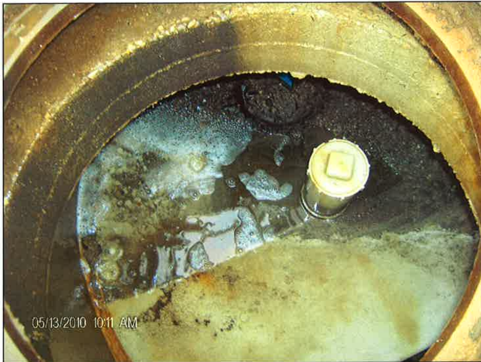
Site Photo 3: May 13, 2010 Stormceptor
