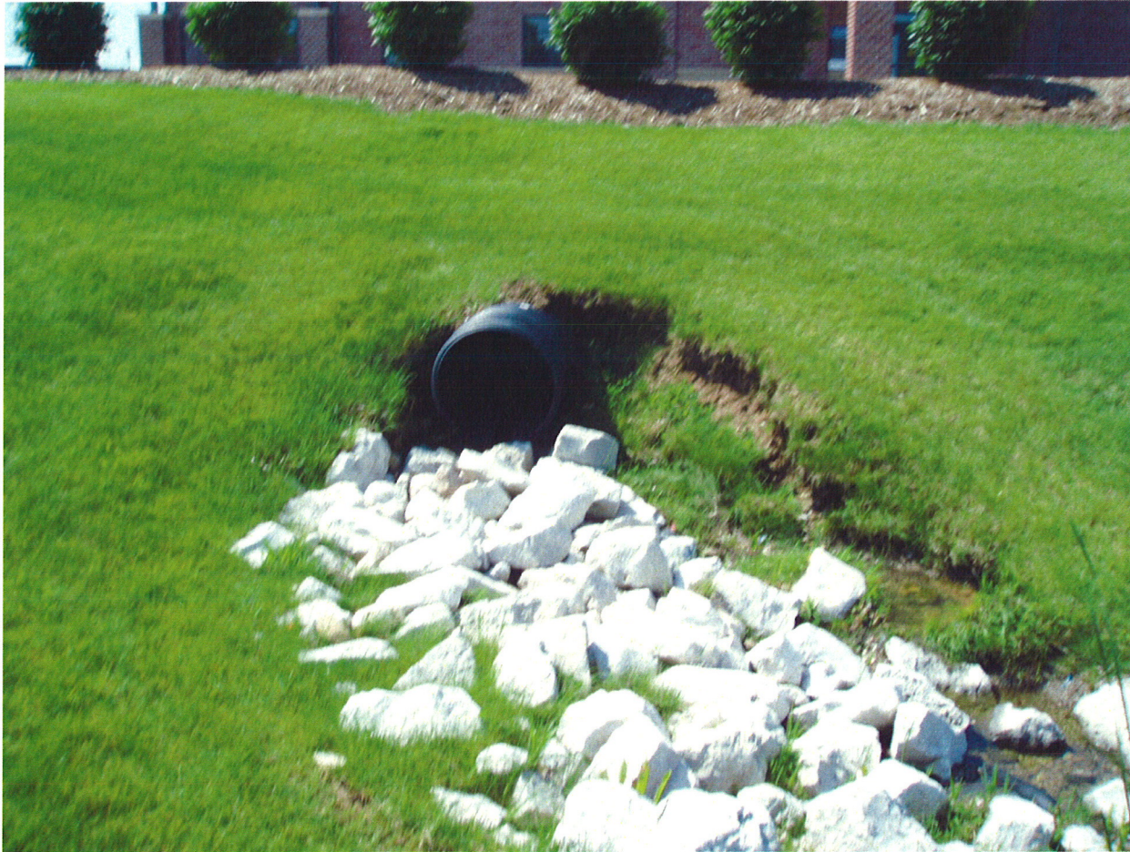
Erosion around southeast inlet pipe.
