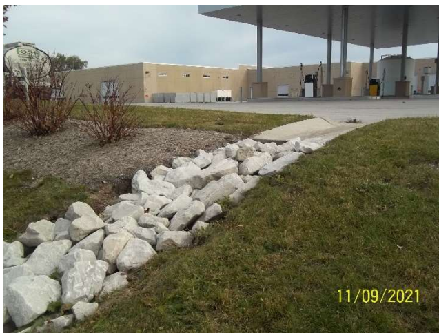
RipRap Parking Lot Drainage
