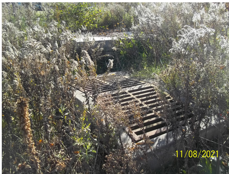
Storm Water Overflow ST015378
