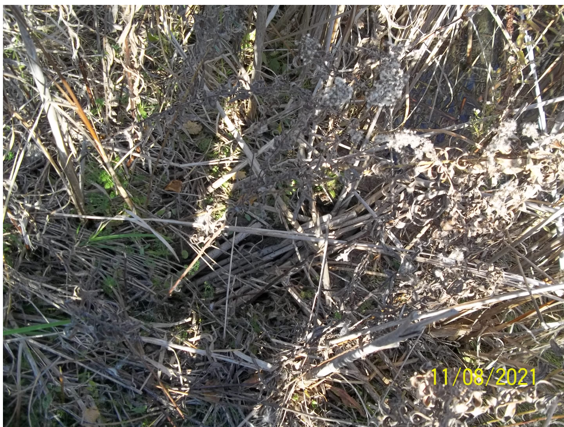
Storm Water Outlet ST015376
