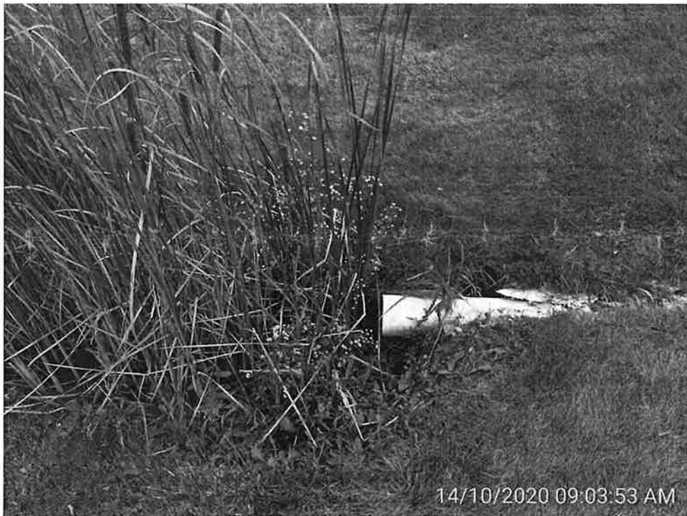
Photo #6: Erosion at 6" outfall pipe
