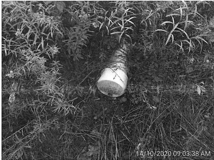
Photo #1: Outlet pipe with 1.6" orifice
