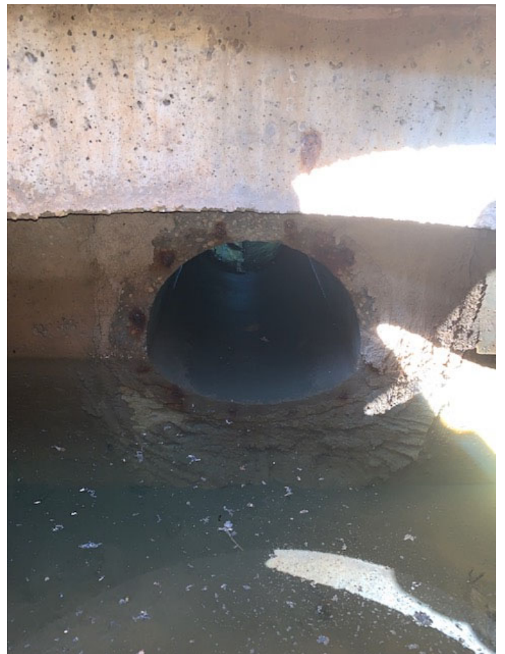
Outlet Pipe from Storage Chamber
