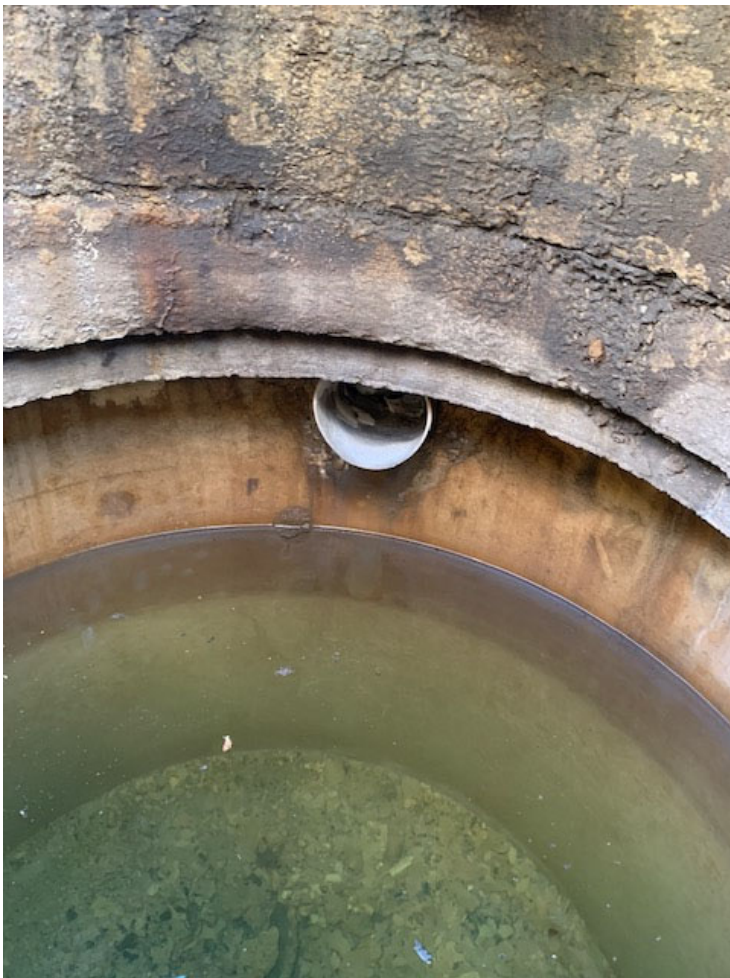
Catch-Basin Connected to Underdrain
