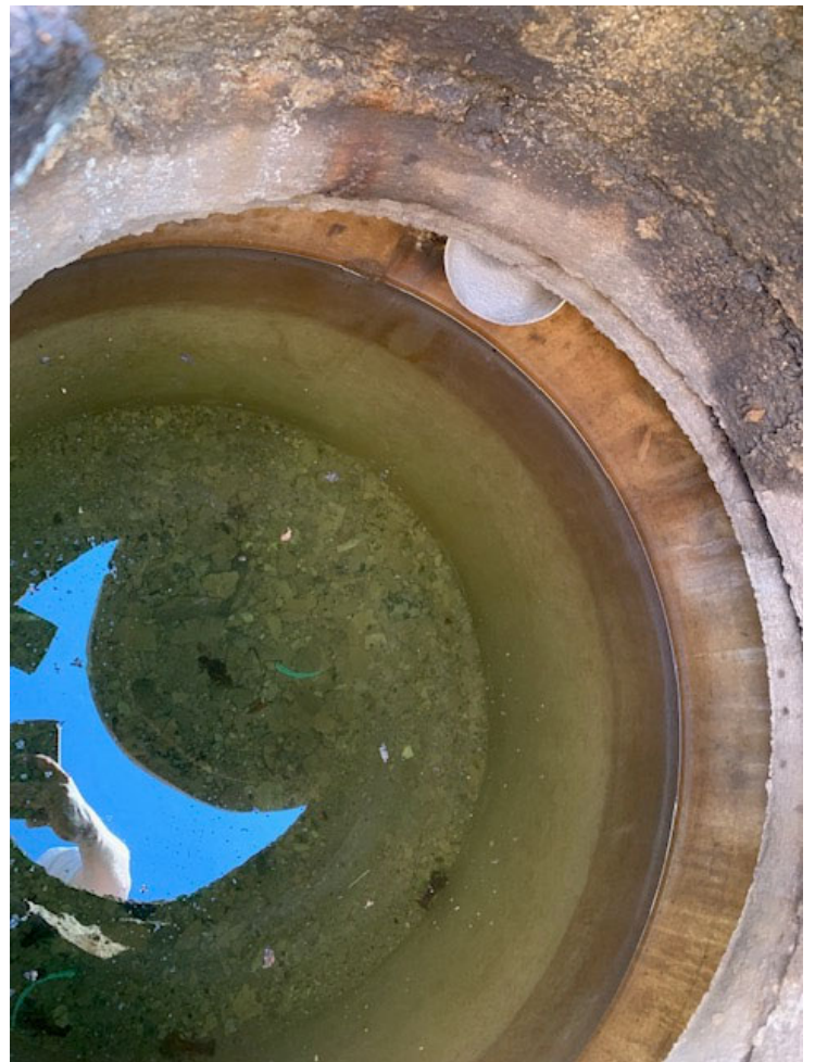
Catch-Basin Connected to Underdrain
