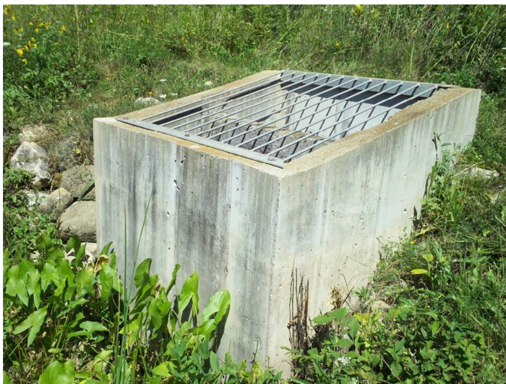
Photo 4: Outlet structure intake silted.
