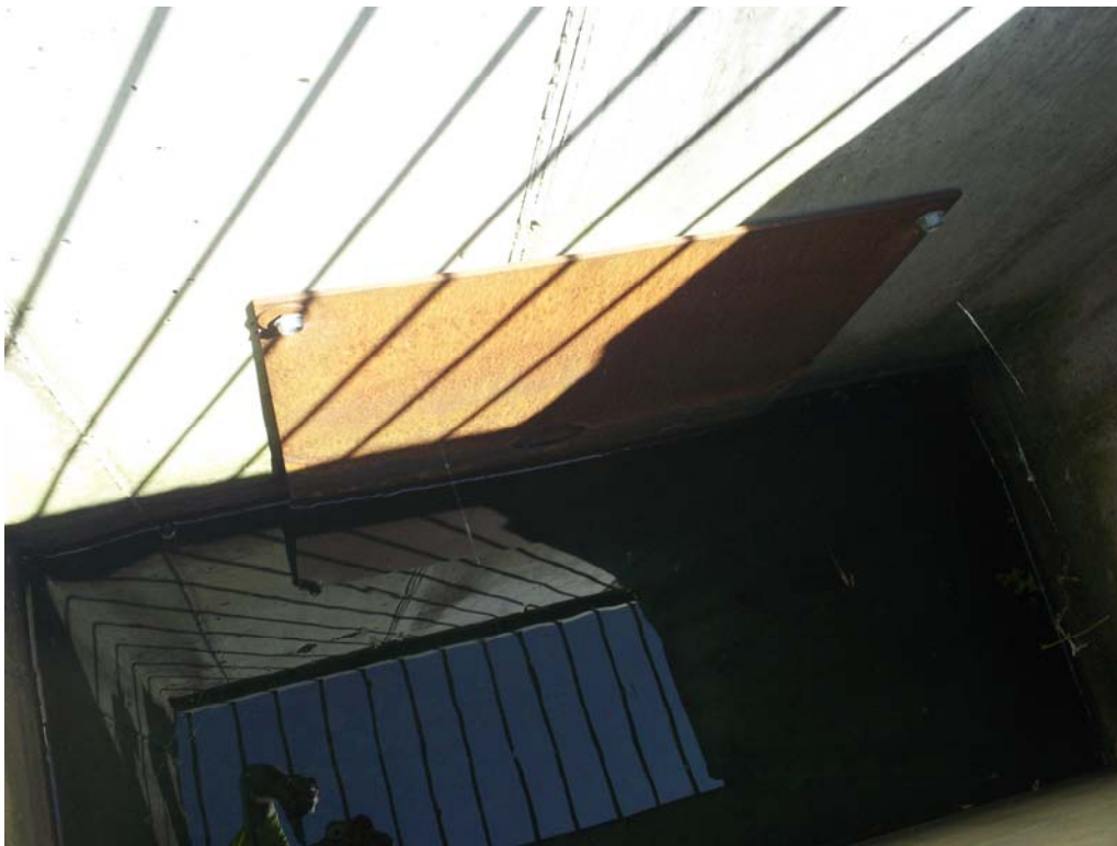
Photo 6: Outlet structure 12" outlet still has the temporary construction plate w/ 4" orifice.
