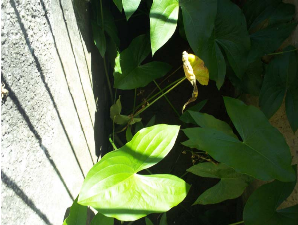
Photo 5: Outlet structure bottom silted and contains vegetations.
