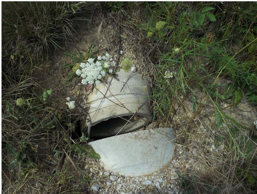
Photo 5: Outfall 3 (ES-8) End section disconnected to pipe.
