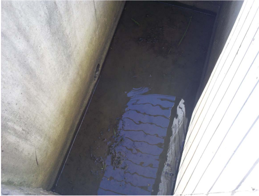
Photo 7: Outlet Structure bottom silted.
