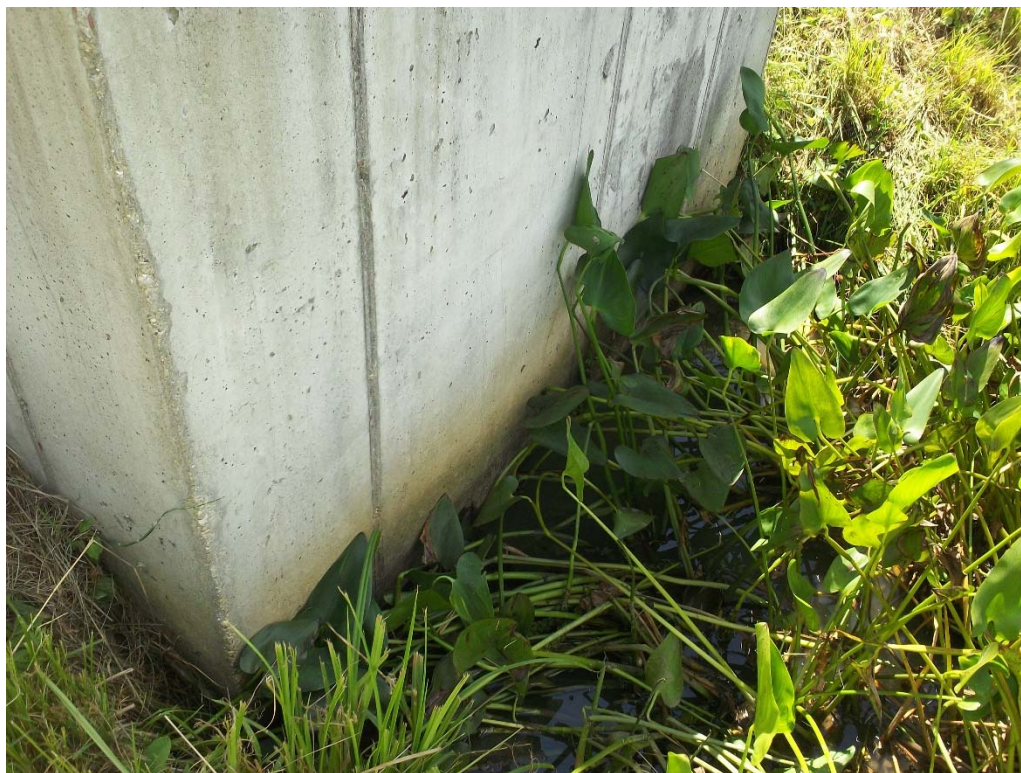
Photo 6: Outlet structure front intake silted.
