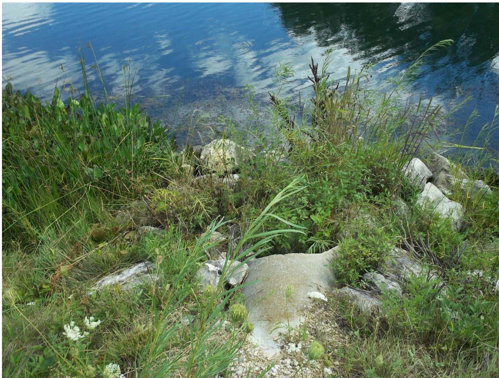
Photo 4: Outfall 2 (ES-7) Erosion at rip rap and heavy vegetation.
