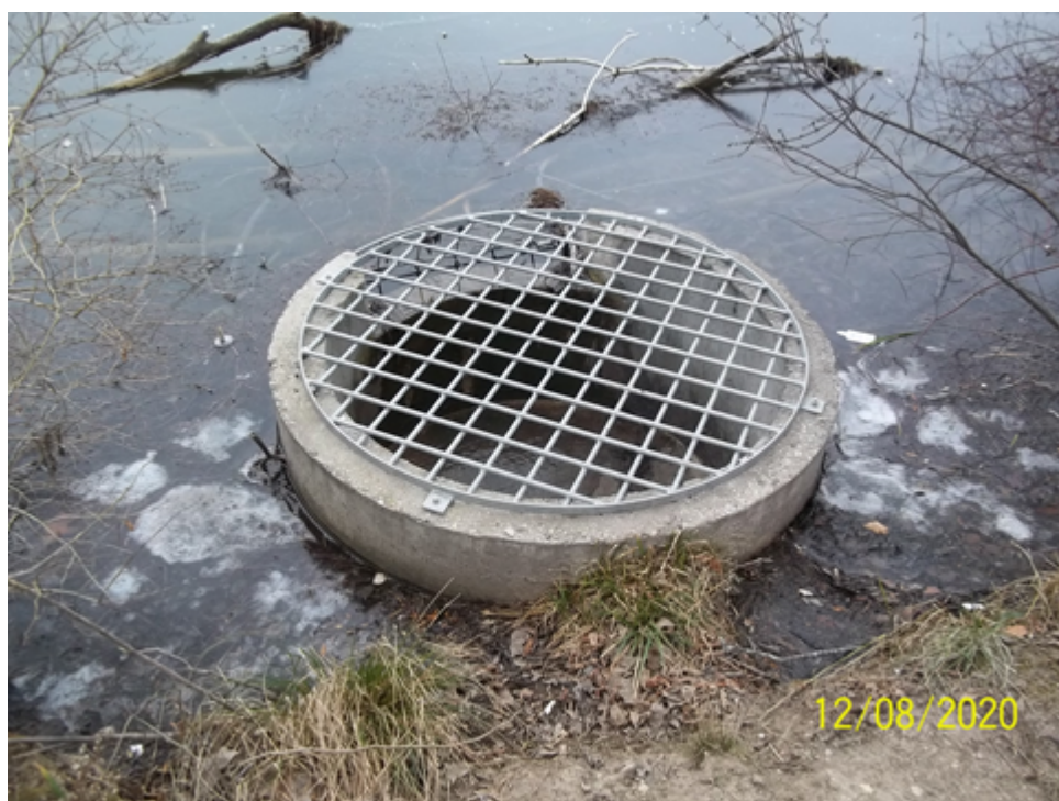
Overflow Manhole ST014271
