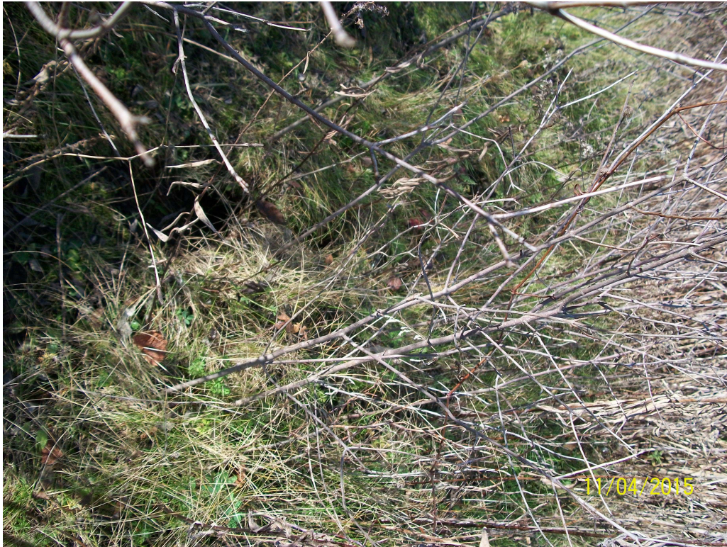
Burrows in N side of SW bank/spillway embankment.
