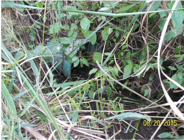
Storm Water Inlet ST010732
